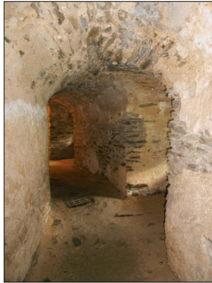
Fig. 4 Casemates of the Červený Kameň Castle built with unworked quarry stone combined with lime mortar (the first half of 16th century) (photo P. Hronček)
